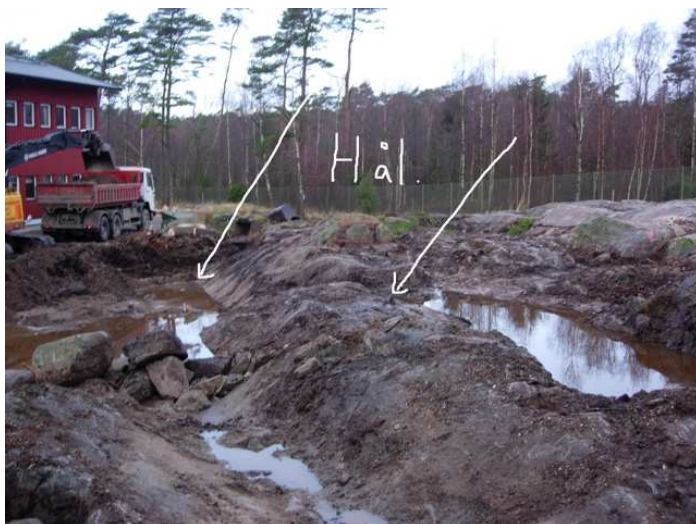
Gravimetry site preparation. Arrows show drill holes "Hål" where cores were retained, and in which ground water level will be monitored. The gravimeter pillars will be erected immediately behind the right arrow after preparation of a flat rock surface. The partly water-filled depression near the truck is in the process of becoming 2.5 m deep until the solid rock surface is touched. The
